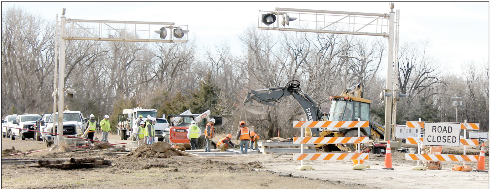
Monarch Cement's railroad project is underway south of the plant in Humboldt. Crews pictured are working on the rail expansion on 1200 Street Wednesday morning. REGISTER/SARAH HANEY
